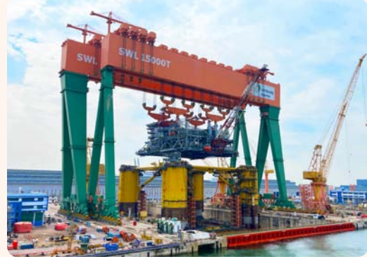
Tandem lift of the Vito RPF mega-topside structure for integration with the FPU hull by a pair of cranes, with combined 30,000-tonne lifting capacity and 100m hook height, at Sembcorp Marine Tuas Boulevard Yard
