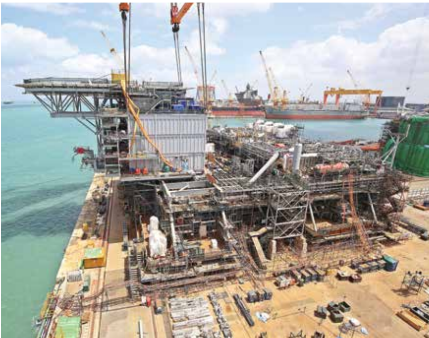
Shell Vito FPU topside and living quarters under construction at Sembcorp Marine Tuas Boulevard Yard
