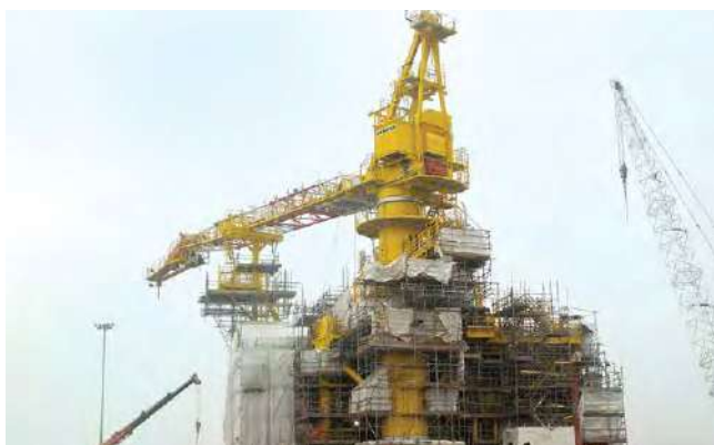
Sembmarine SLP is constructing a power generation module for Maersk Oil's Culzean field
